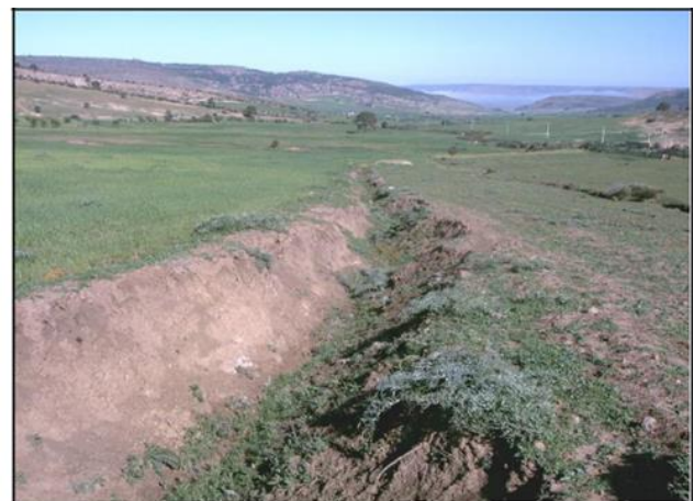
Photo 2. Erosion in ditches in lowland areas (Aouadj, 2022)
